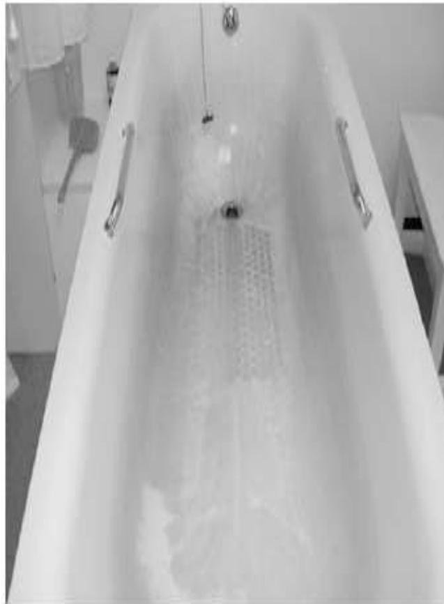
Figure 4. Staining as a result of Silver / Copper ionisation
